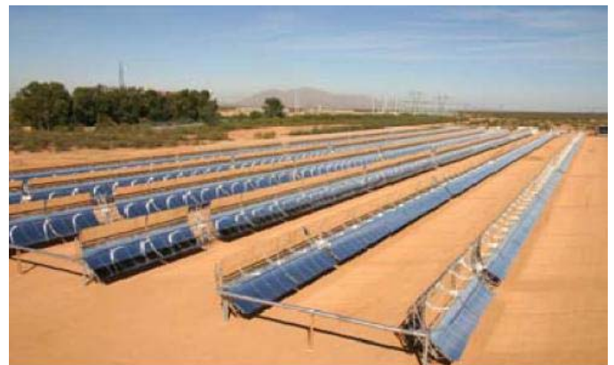
APS Saguaro 1MWe solar power plant
